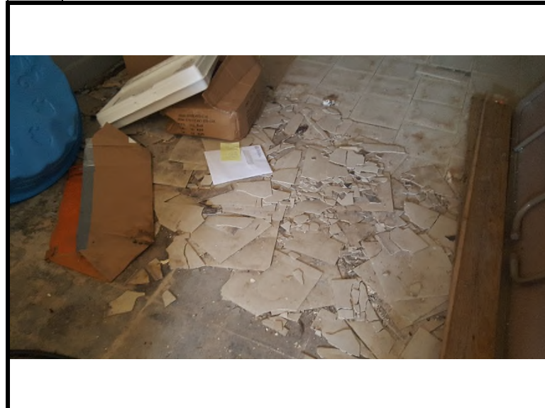
4 The 12-inch tan vinyl floor tiles and associated black mastic in the basement hallway tested positive for asbestos (5% & 2% chrysotile). The floor tiles are considered to be damaged.
