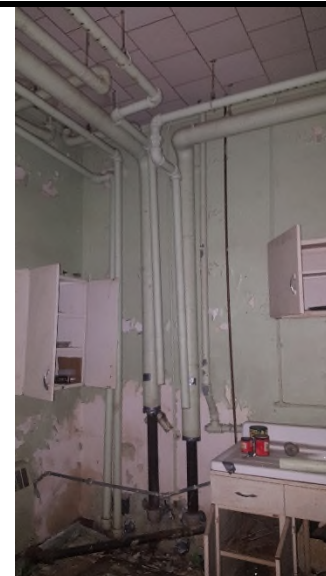
8 The hard joints in the basement piping contains 70% chrysotile.
