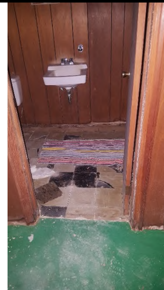
6 The green 9-inch vinyl floor tiles and black mastic in the teacher's restroom in the basement tested positive for asbestos (3% & 3% chrysotile).
