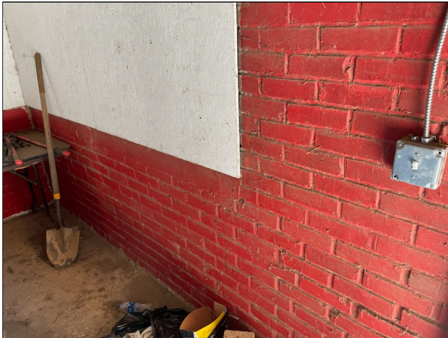
6 - Red LCP on Interior Brick Walls in South Barn
