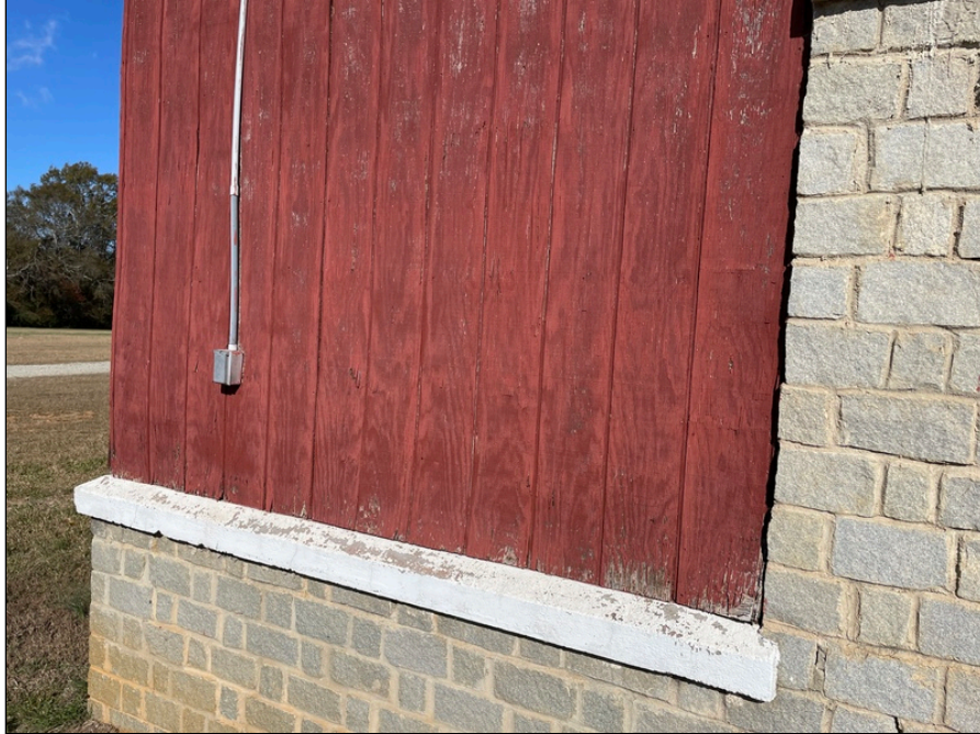
5 - White LCP on Concrete Trim of South Barn
