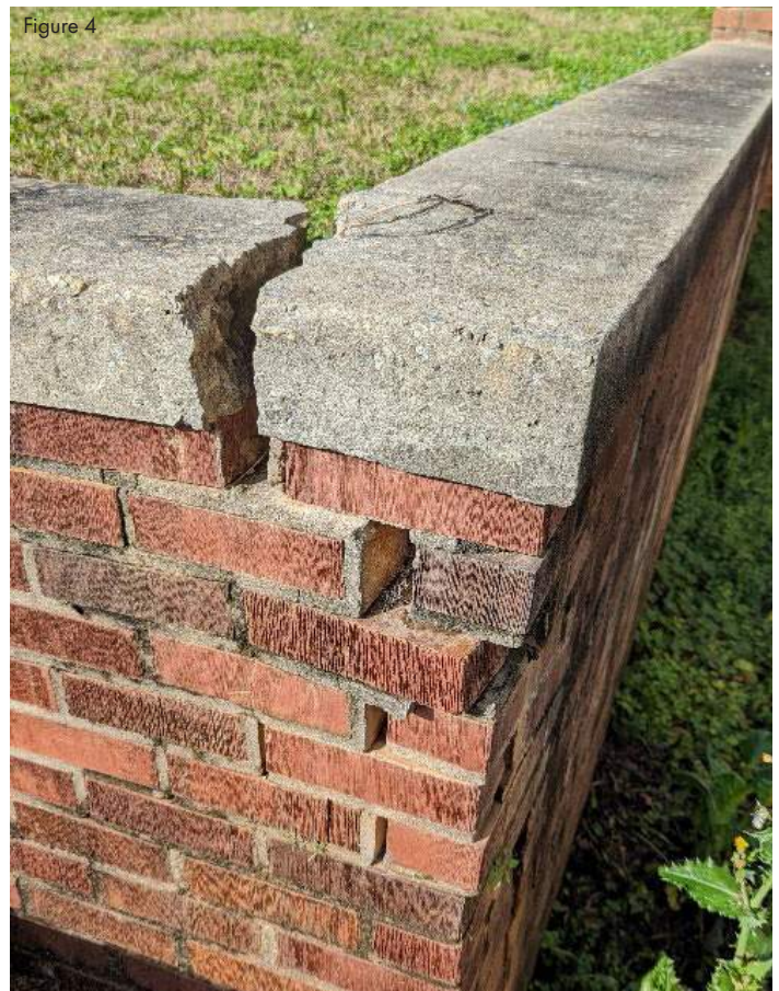
Masonry retaining wall failing
