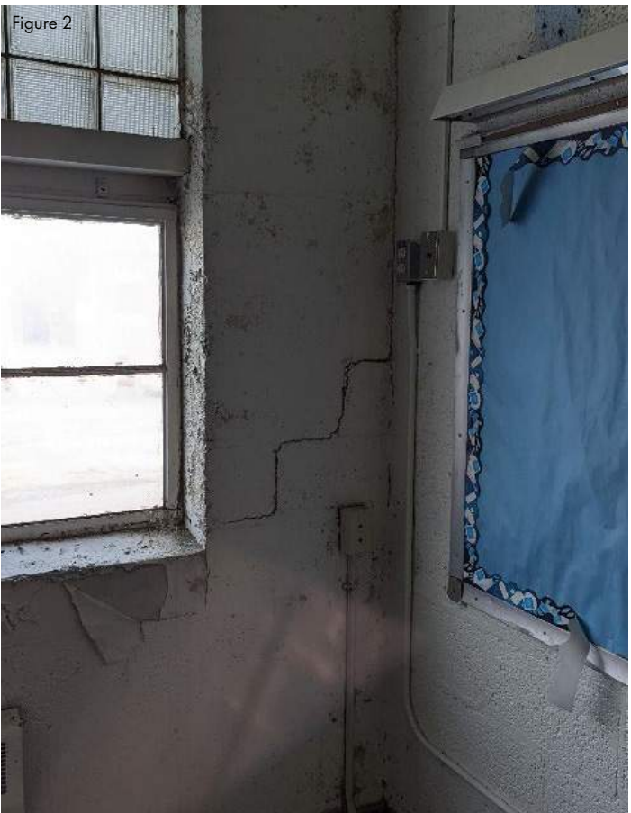
Front wall cracking and indication of moisture intrusion
