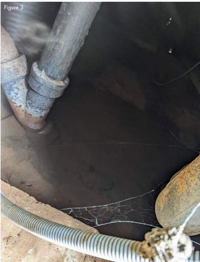
Standing water in crawl space
