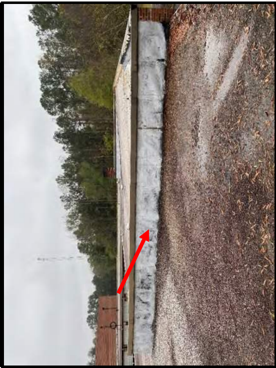
11 Silver sealant on parapet walls tested (<1% chrysotile) PLM analysis and no asbestos detected by TEM.
