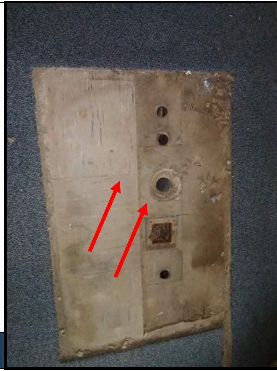
3 12-inch dark tan vinyl floor tile and black mastic and 9-inch brown vinyl floor tile and mastic tested positive for asbestos (3% chrysotile).
