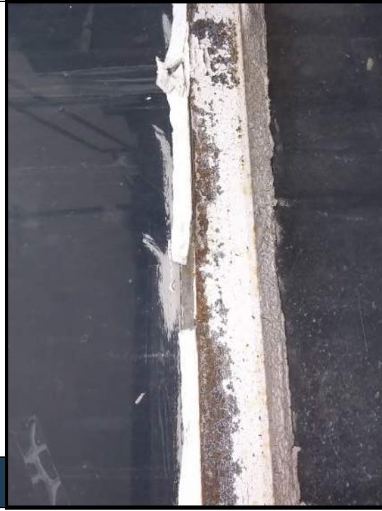
4 Window glazing tested positive for asbestos (2% chrysotile).
