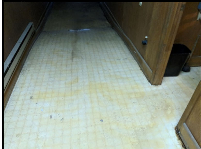
8 The tan linoleum located in the south side of the garage building tested negative for asbestos.
