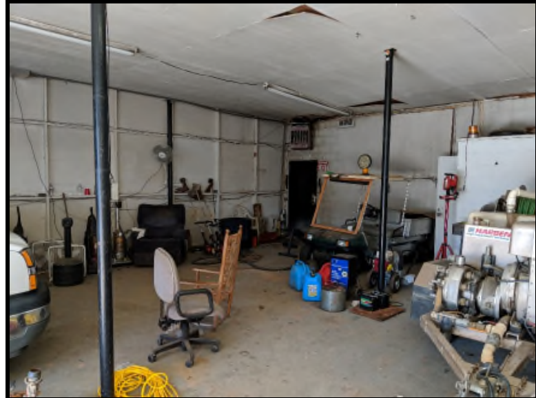
6 Typical interior view of the garage building attached to the Town Hall.
