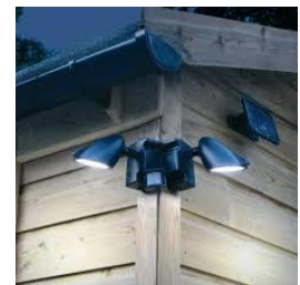
Exterior Security Lighting
